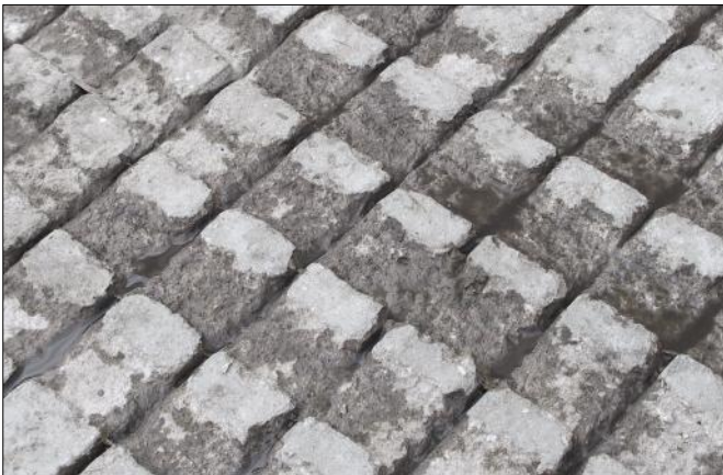
Figure 5. Rough surface due to floor degradation. Could result in very high point loads in solar corium.
